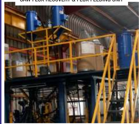
SAW FLUX RECOVERY & FLUX FEEDING UNIT
