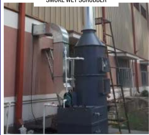
SMOKE WET SCRUBBER
