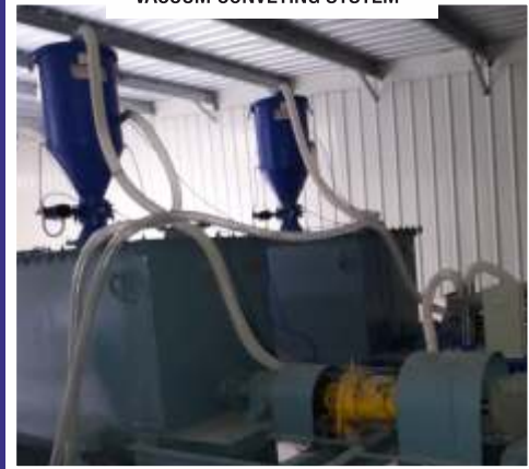
VACUUM CONVEYING SYSTEM
